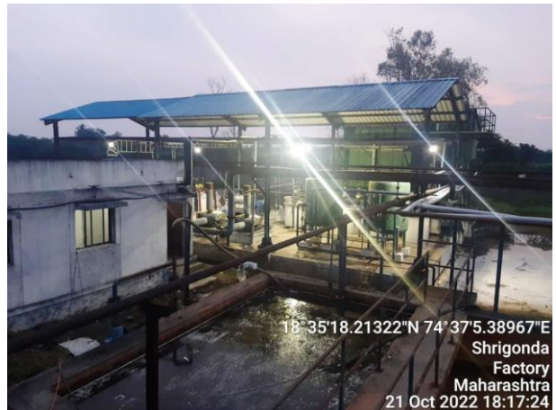
Photograph-6: CPU of distillery unit ETP.
