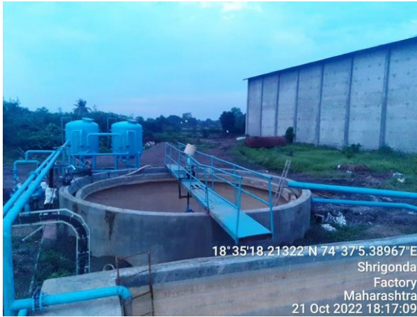
Photograph-7: CPU of sugar unit ETP.
