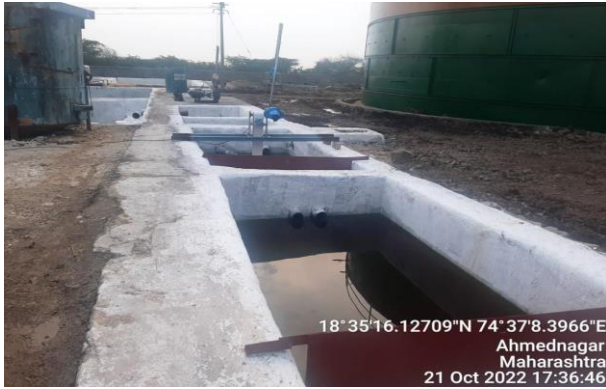
Photograph-1: Grit chamber and oil & grease skimmer installed at ETP.
