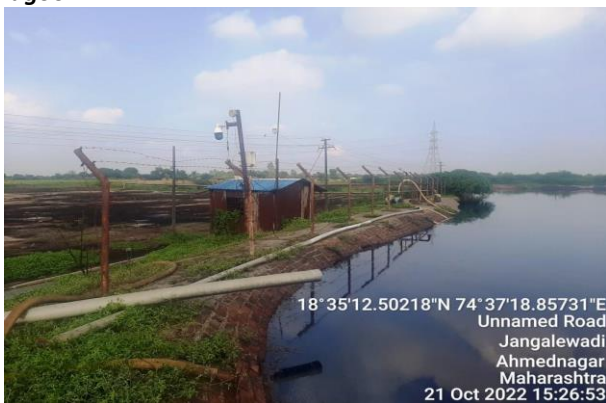
Photograph-11: PTZ camera installed at bio-compost yard of distillery unit.
