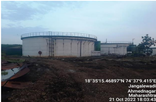
Photograph-3: UASB reactor of distillery unit ETP.
