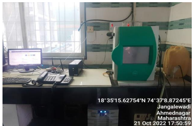
Photograph-12: OCEMS installed at final treated effluent conveyance pipeline of sugar unit ETP.
