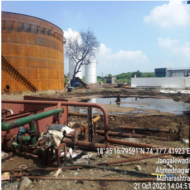
Photograph-13: A view of area where molasses storage tank blast occurred.
