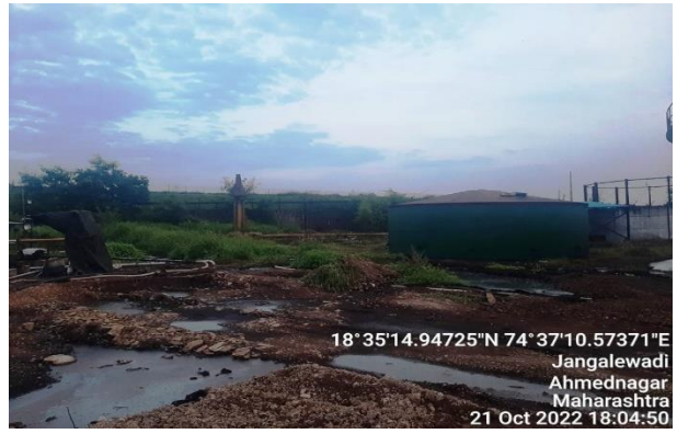
Photograph-4: Biogas holder and flaring system.
