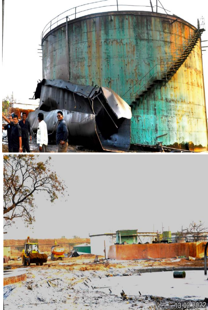
Figure 2.2: Photographs of the damaged area
